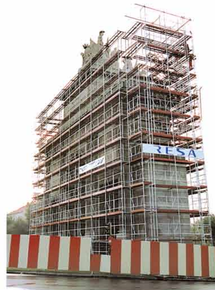
Scaffolding for the integral rebuilding of the Gate of Toledo, Madrid, Spain
